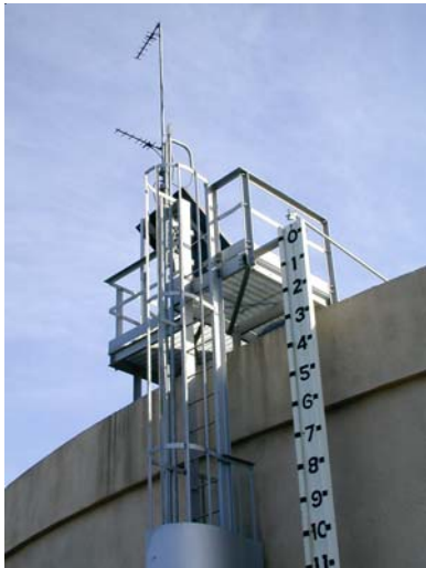
Wireless solar-powered Tank Level Monitoring
